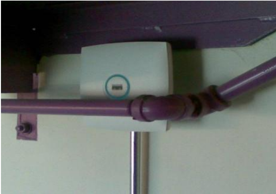
Ceiling mount AP mounted on the wall up against metal pipe (poor coverage)
